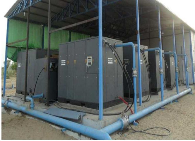
Figure 3: SIAD TEMPO 2 1500 high pressure compressors
