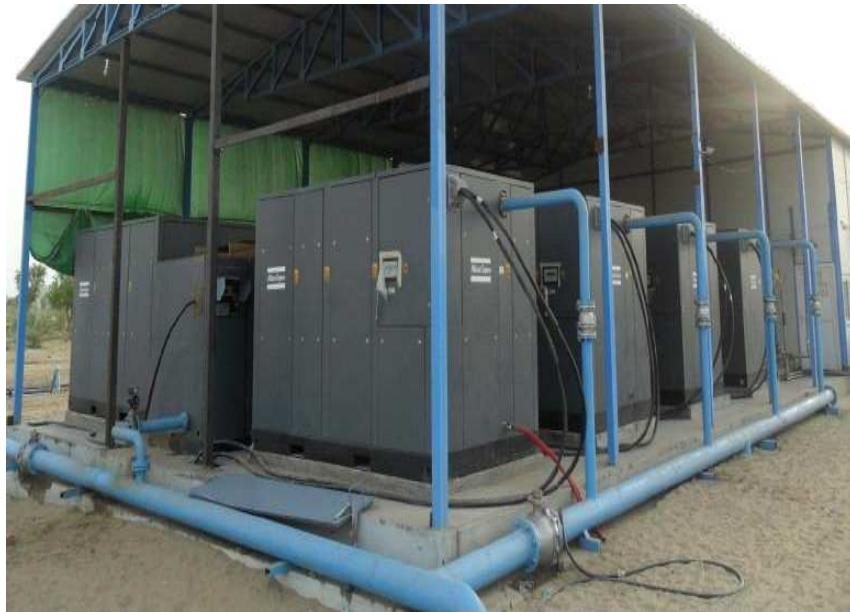
Figure 4.2: SIAD TEMPO 2 1500 high pressure compressors
